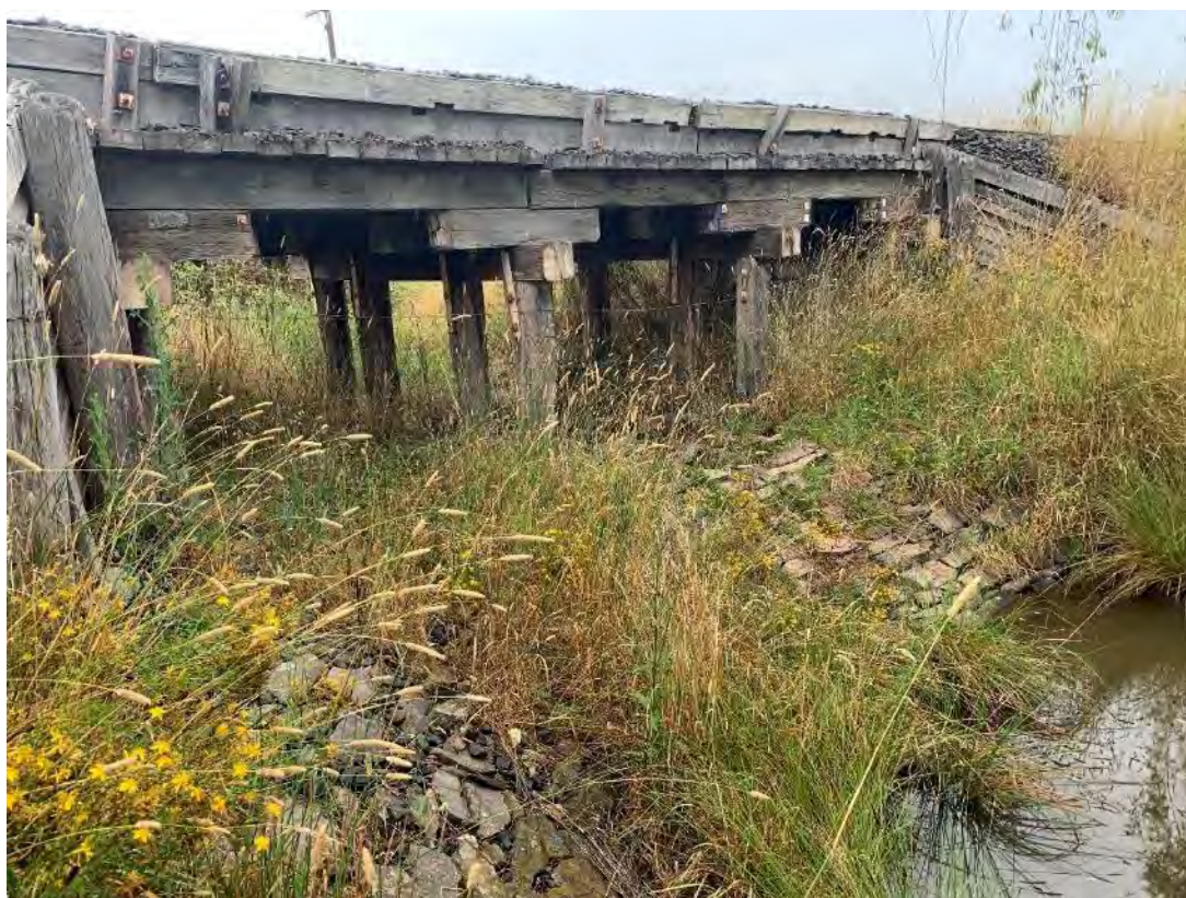
Figure 5-1: The top image shows a general view of the minor 10m Bridge from an abutment. The timber girder under bridge consists of 3 spans of 3.3m. Each bent consists of 4 driven timber piles and a single headstock. Headstocks are attached to the piles using a vertical steel bracket on either side. Note kerb support completely split vertically through middle.
