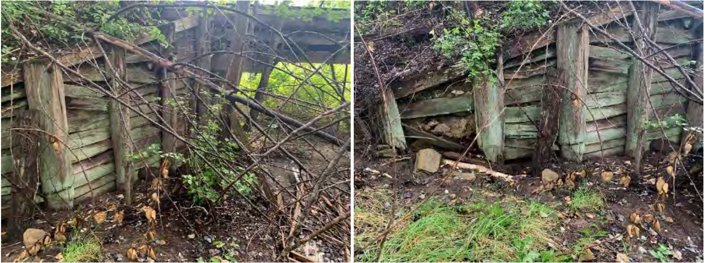
Figure 4-8: The timber wingwalls have undergone significant deterioration with timber sheathing completely rotted and failing in several locations. Due to this the walls' ability retain the approach fill material is poor leading to erosion and excessive loading.
