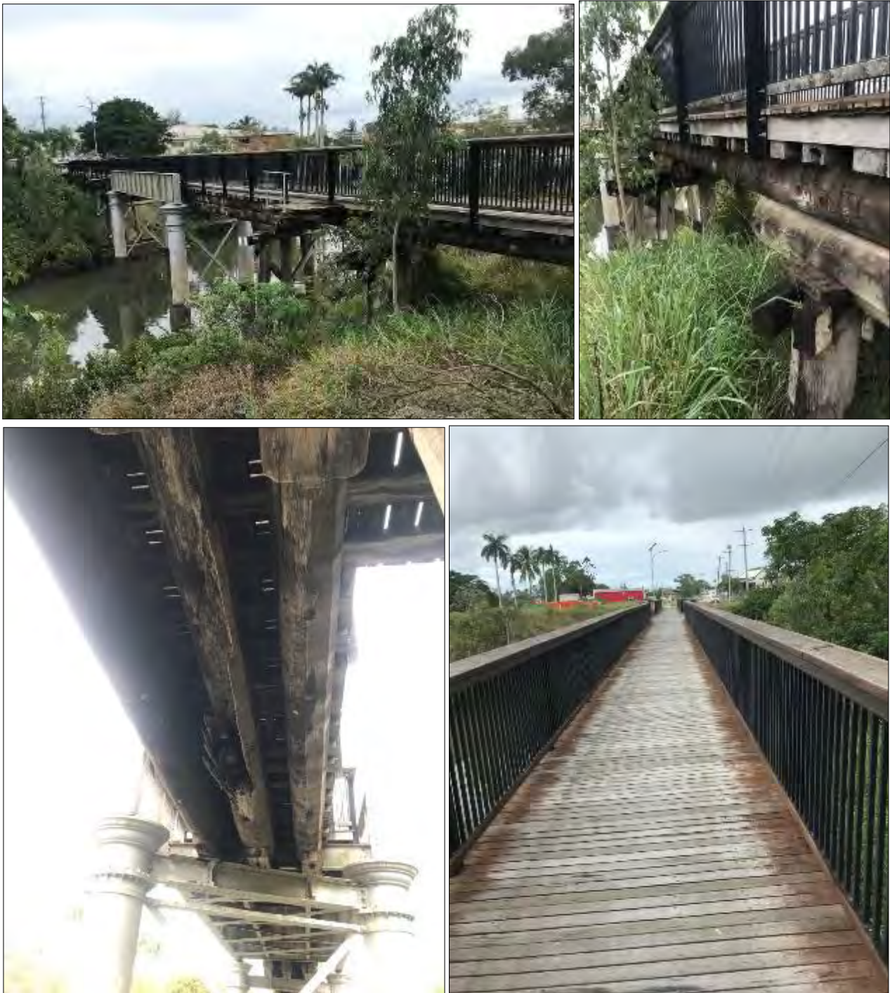
Figure 12-2: The above photo series demonstrates a similar repair to Option 1 type of refurbishment (build off existing railway bridge) used for the construction of a pedestrian bridge in Bundaberg CDB. The existing railway bridge was left un-touched and a new hardwood deck system with handrails was installed. Six 100mm x 250mm timber joists were placed on top of the existing transoms (rail ties) with a 38-50mm thick hardwood deck installed on top. This option will likely be the lowest cost but also carries the shortest expected lifespan. As seen in the bottom left photo above, one of the girders has failed and fallen out creating a ‘weak’ point along the bridge. Due to a high residual capacity of timber and the continuous joists, a complete failure of the bridge (span) hasn’t occurred yet but is only a matter of time unless extensive maintenance is undertaken.
