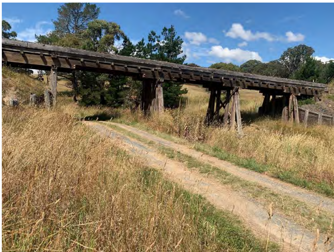
Figure 8-1: General view of Deep Creek Bridge from abutment 1 looking towards abutment 2. The timber bridge is 5 spans long and approximately 32 metres in length (Spans 1 & 5 – 4m and spans 2, 3 and 4 – 8m). Note span 2 passes over the road (4.2m Clearance) and span 3 passes over a creek 2m wide and 0.5m deep.
