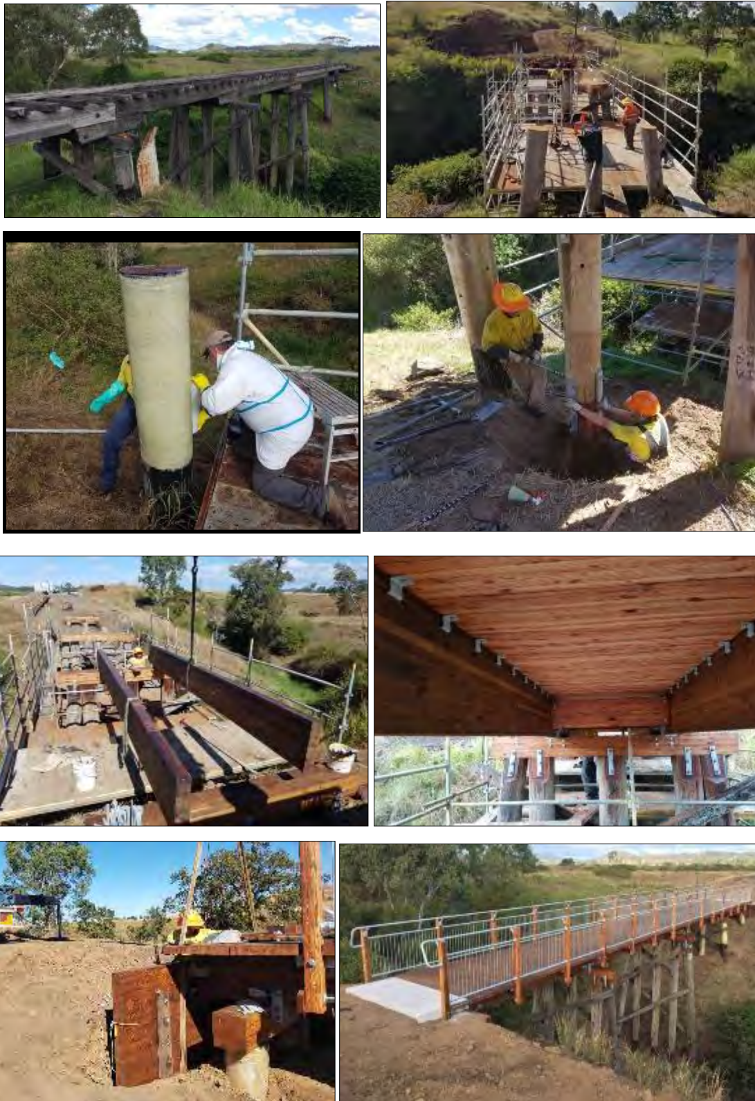
Figure 12-4: The photo series above demonstrates Option 3 type of fix that was completed on Jimmy Gully Bridge along the BVRT. The existing poor condition superstructure was removed, and the piles were repaired with high strength fibre or posted with new section. New glulam back wall, caps, girders and deck system were installed utilising a horizontal connection detail.
