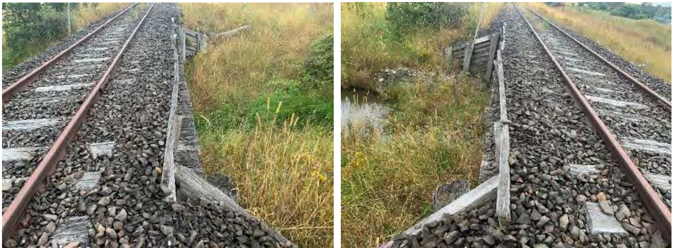
Figure 5-7: View of both ballast tray side walls. Both side walls were found to be in fair to poor condition, with minor deterioration of sapwood present at all lengths. Photo on the right shows the side walls support leaning backwards creating a deformation in side wall length. Photo on the left shows a significant bow in middle length due to bearing the load from the rock ballast.
