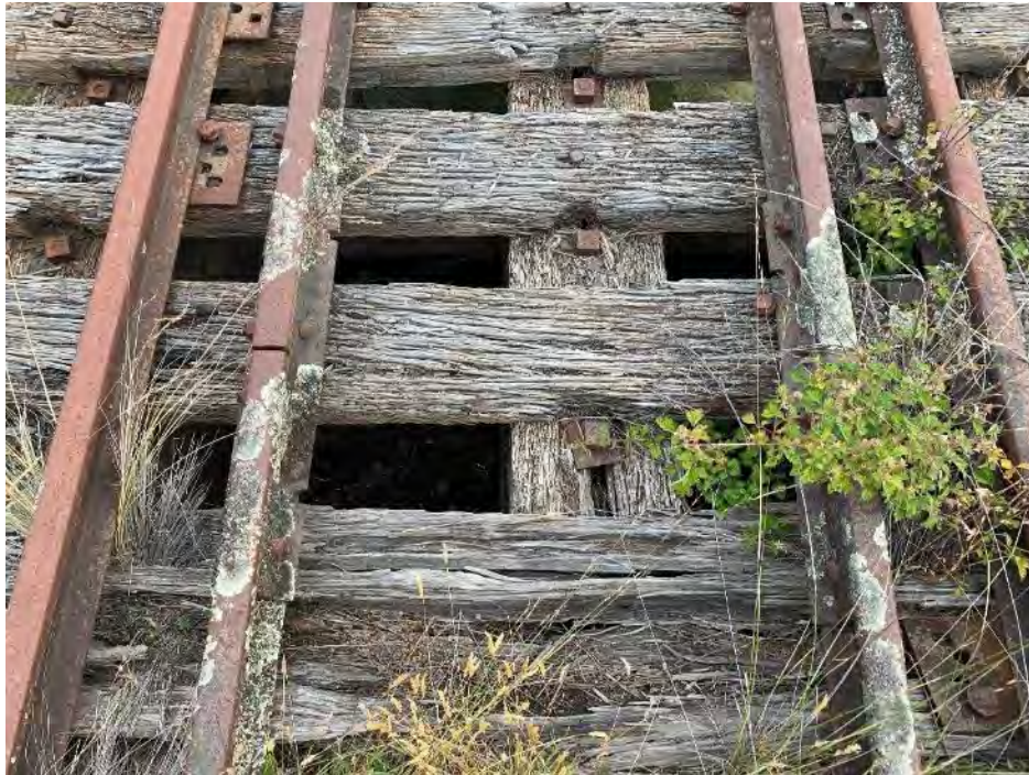
Figure 11-7: View of the bridge open deck, transom sleepers were found to be in poor to very poor condition with significant decay, cavities and severely damaged members present throughout. It was noted that the vertical connections to the top girders were seen to funnel moisture and increase the moisture content present in both elements causes significant decay. When the moisture content exceeds 22%, timber consuming fungi are activated, and the decay process begins. Top girders were found to be in poor to very poor condition.
