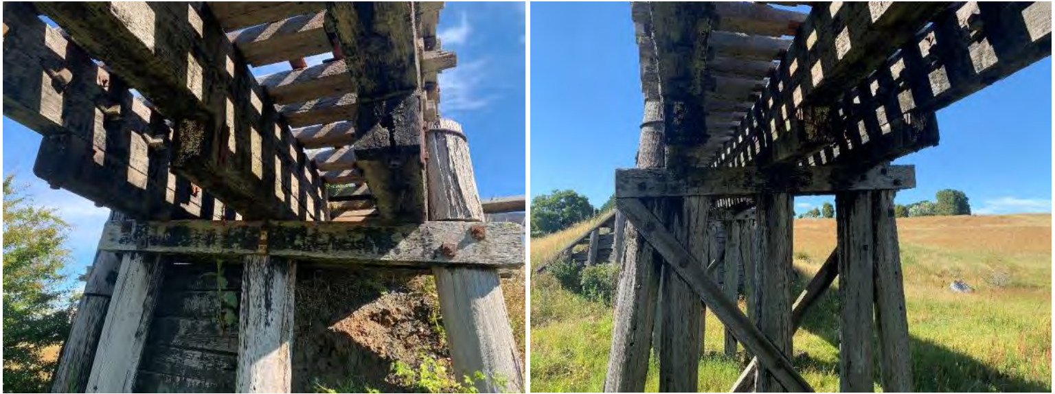
Figure 9-3: The images above show the substructure configuration. It is seen that double stacked girders have been used in addition to split headstocks and corbels. Both images show significant water stains and decaying of corbel ends. The left image identifies a large cavity present in the end of corbel 1 AB1. It was noted that AB1 sheeting has failed.
