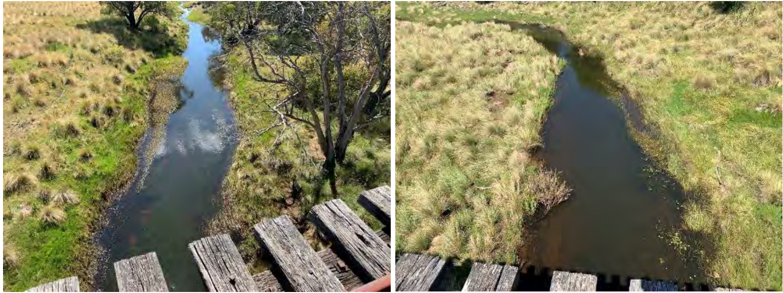
Figure 10-9: Left side image shows the view looking upstream and the right-side image shows the view downstream of the bridge of the edge of the open deck bridge.
