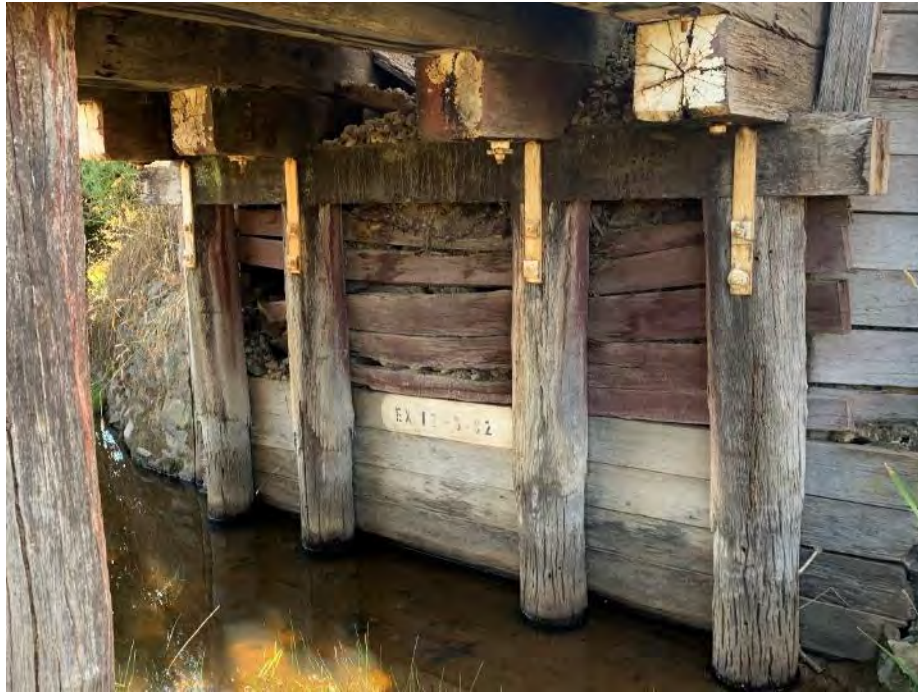
Figure 6-4: General view of Abutment 1 shows the timber sheeting in very poor condition as top half is failing and backfill material is eroding. Note: Hole in decking above abutment causing significant material loss from rock ballast above.
