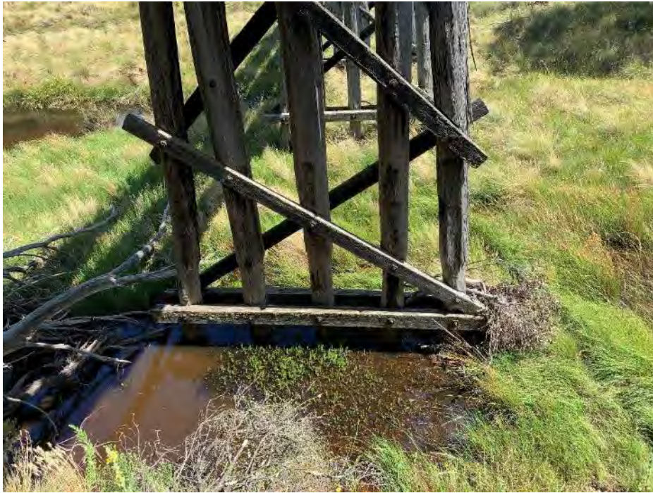
Figure 10-3: Significant decay is present on all piles in above image. Large decrease in pile cross-section on the bottom end of the piles located in the river (Body of water). Debris is caught up in the wales and surrounding areas of pile bents. It is recommended that deteriorated sapwood be removed appropriately.
