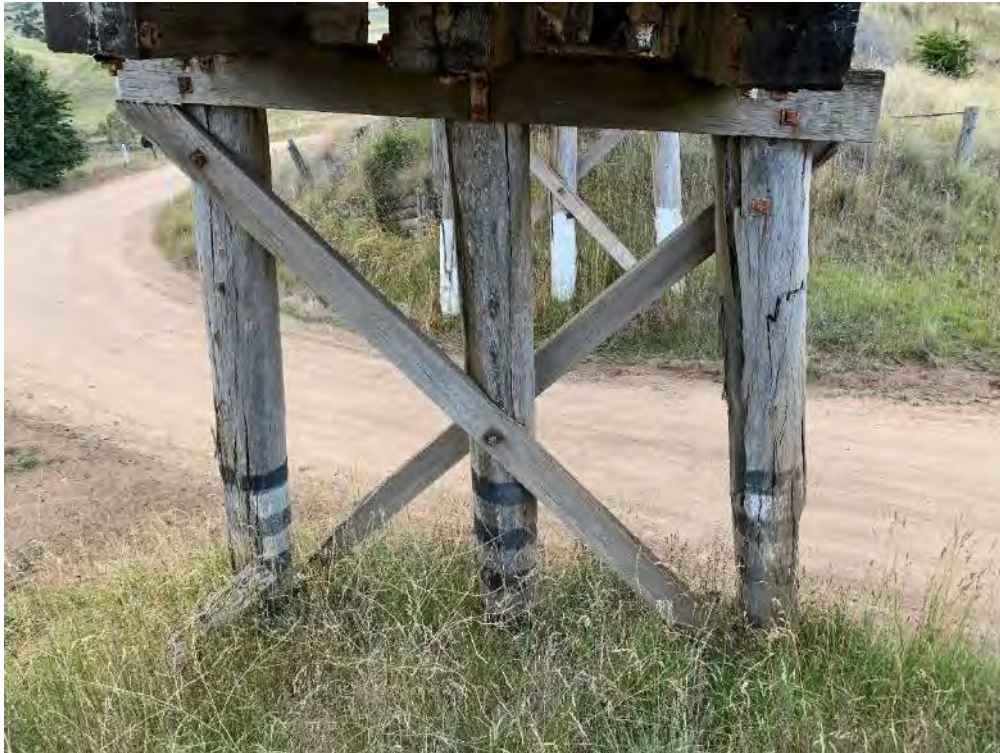
Figure 11-3: General view of pile bent 2. piles were found to be in poor condition. With significant sapwood decay present in all piles, it was noted that all piles have large vertical splits through the horizontal connections. The bottom sections of the timber piles were determined to be a ‘hotspot’ for decay due to increased moisture retained by the overgrown vegetation.
