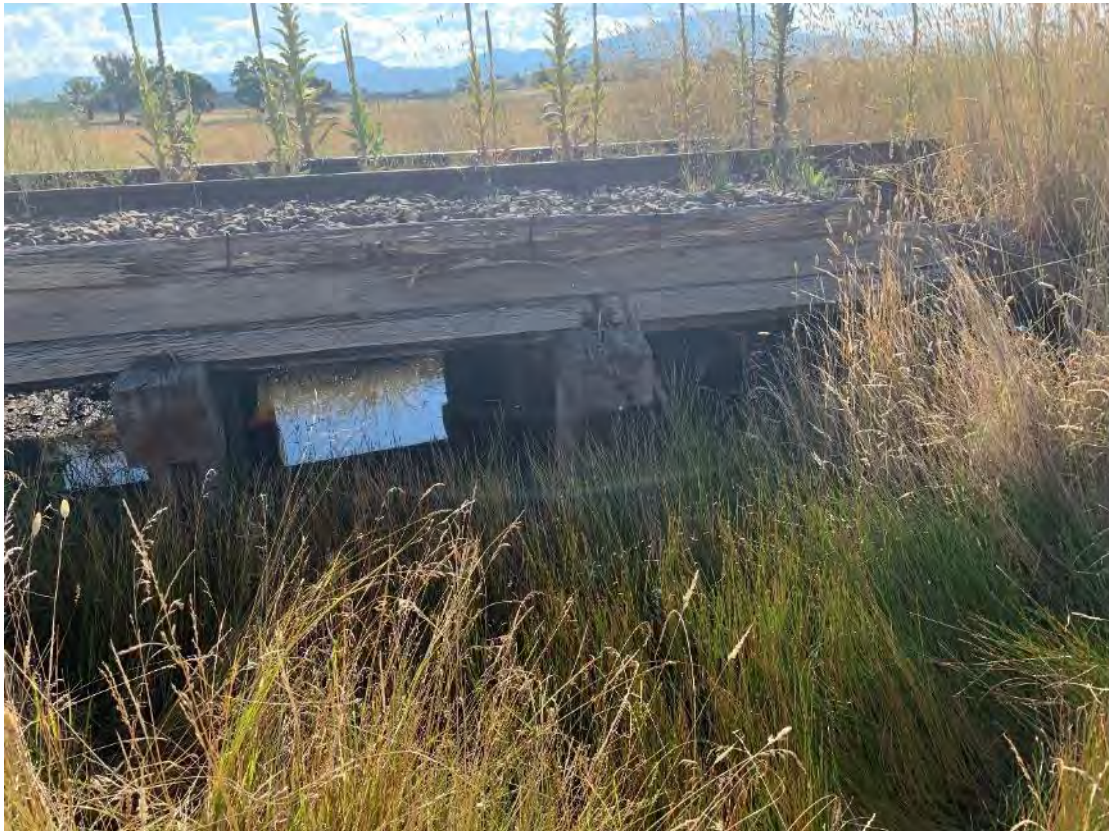
Figure 7-1: The image above shows a general view of the 7m minor bridge (Williamsdale Rd). The consists of 3 spans each span is 2m in length, substructure includes 2 pile bents and 2 abutments that each have 4 driven piles, a pile cap and 4 girders. At the time of inspection there was water approximately 0.5m deep in Spans 1-3. There is a large amount of vegetation growth around the substructure which keeps the moisture content high in the timber. When the moisture level in the timber is above 22%, decay-causing fungi can start to grow; when the moisture content drops below this level, the fungi become dormant, and decay will be arrested until the moisture content rises again.
