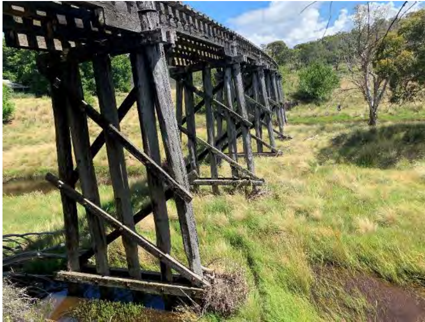
Figure 10-7: Above image shows the left curve and camber in the bridge. The bent configuration is also highlighted, it was noted that significant overgrown vegetation and debris build up was present at the base of all bents. This increases moisture retention leading to accelerated decay of the lower timber elements.
