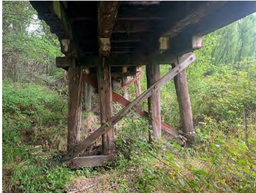
Figure 4-2: View of the typical timber pile bent configuration. The bent is comprised of 4 driven piles, single timber head stocks and corbels. The bent is also supported by a double cross bracing system with sashes at halfway and timber wales at the bottom. Overall, the timber bents were found to be in a poor to very poor condition. Note the surface brown rot fructing bodies on the faces of some of the cross braces -orange brown colour.
