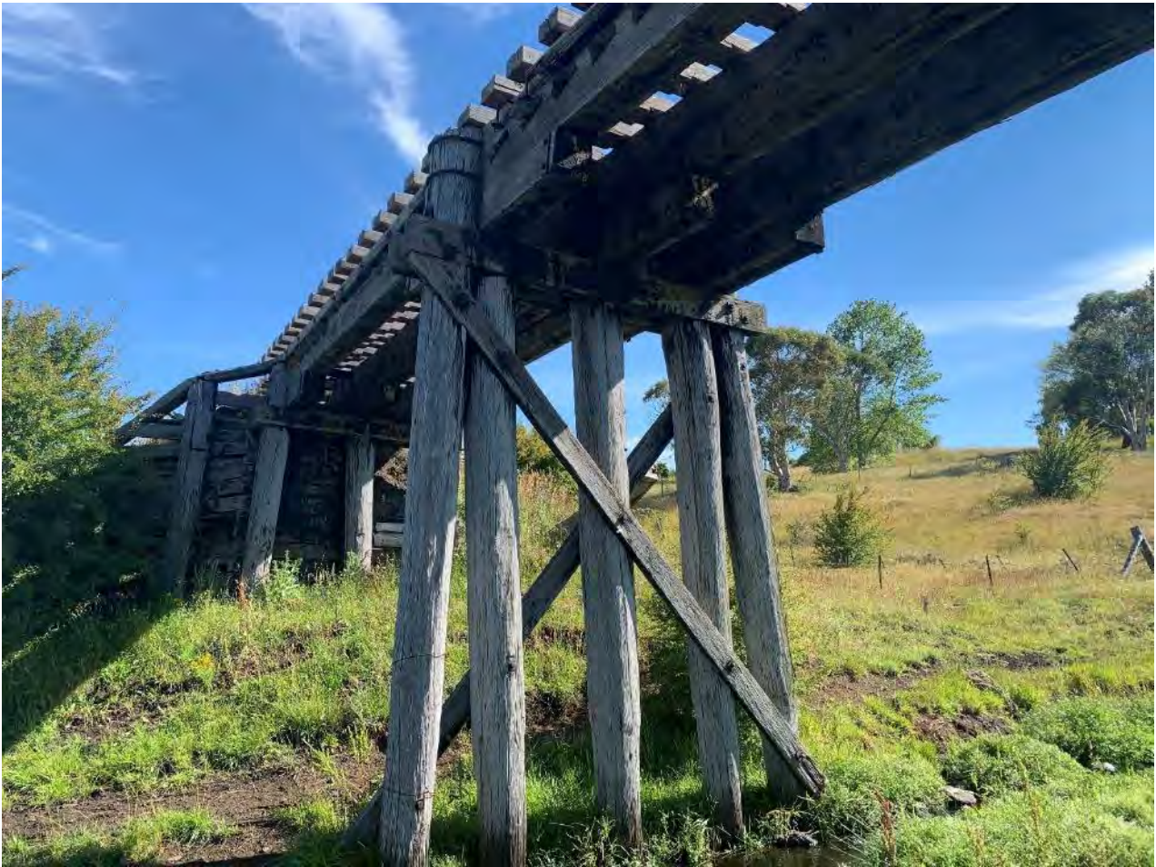
Figure 9-2: View of the timber pile bents configuration. PB 2 and 3 comprise of 5 driven piles (3 Plum piles directly under the girders and 2 batter piles on either side). Pile bent 2 and 3 are supported by cross bracing. The two abutments do not contain the cross bracing and are support by timber sheeting to retain backfill. It was noted that the bottom section of several posts has started to undergo decay. This can be expected due to the timber posts being exposed to increased moisture in overgrown vegetation, debris, and the nearby creek. Once the moisture content in the timber elements reaches 22%, decay causing fungi are activated and the decay process begins. Overall, the timber bents were found to range from poor to very poor condition.
