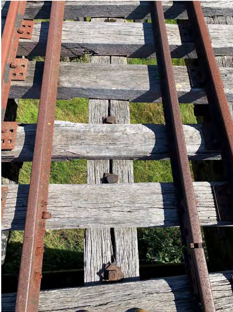
Figure 9-8: Top view of bridge surface, found to be in poor to very poor condition due to major vertical crack through the middle girder and major decay present in all other girder lengths. Vertical connections expose the bright wood to weathering and funnel watering, this leads to accelerated decay and higher moisture content. Transoms appear to be in fair to poor condition with no major decay or defects present. Note the smaller guard inner guard rail on this open deck railway bridge
