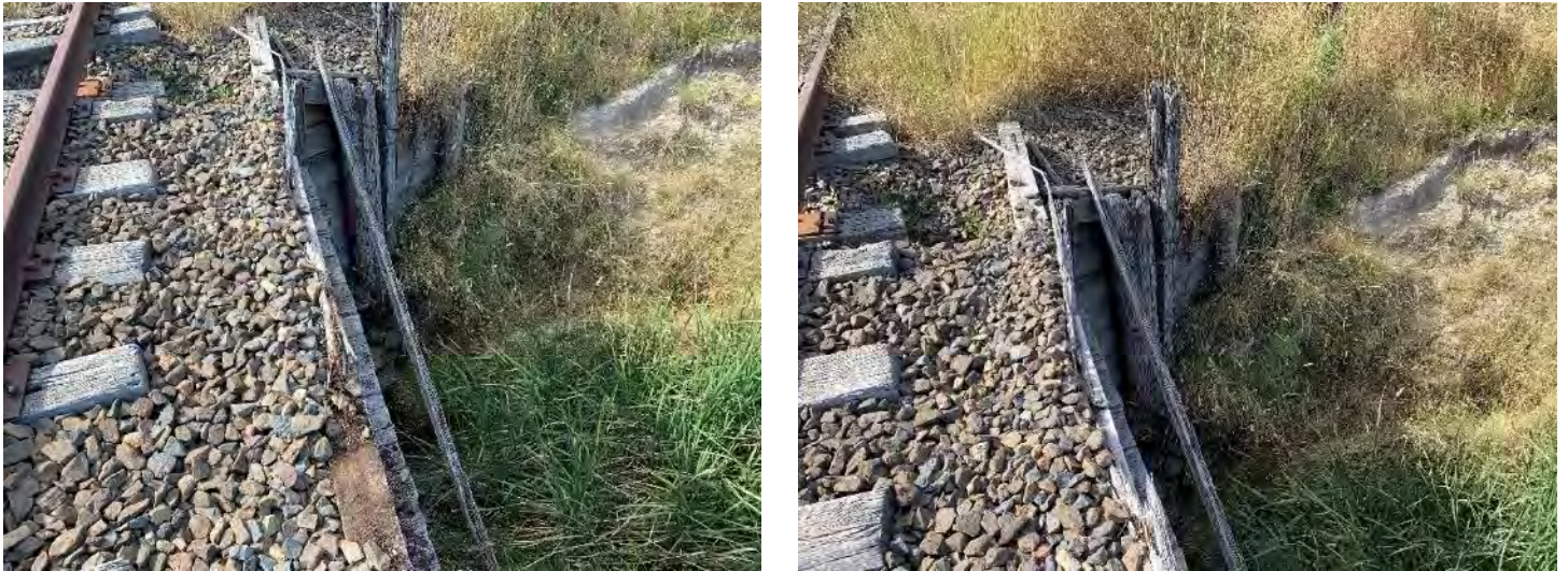
Figure 6-8: View of timber ballast tray side walls, spacing between side walls was 3.5m. Side walls were found to be in very poor condition with significant rot and decay present.
