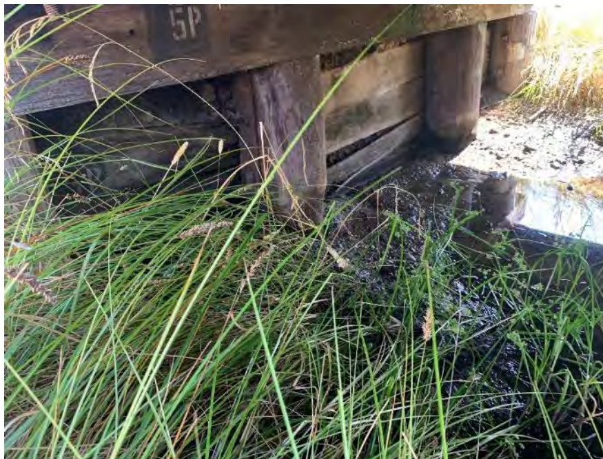
Figure 7-3: View of abutment 2, overall, in a poor condition. Sheeting planks have separated due to spiking to the pile backs in the breast wall, causing loss of fines in the approach fill material through gaps.
