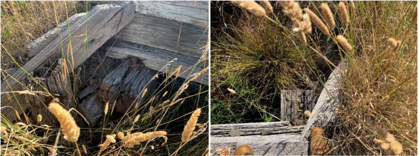
Figure 7-4: Top view of abutment cap connection. Cap is in very poor condition; severe deterioration is present in the ends and at the vertical connection. When a vertical connection is not sealed appropriately it exposes the heart wood to excess moisture accelerating decay. As seen in the photo a large crack is present at the end and a cavity is present at the top of the vertical connection.
