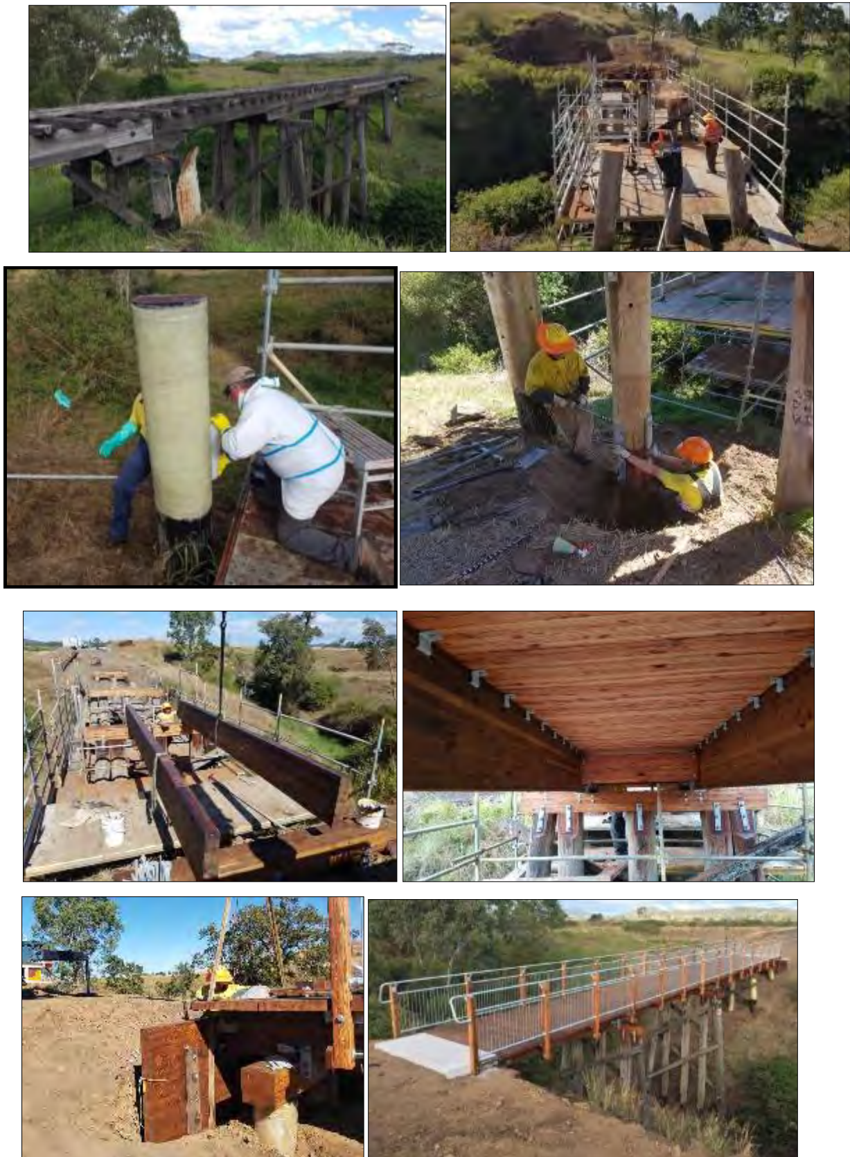
Figure 12-9: The photo series above demonstrates an Option 2 type of fix that was done for Jimmy Gully Bridge along the BVRT. The existing poor condition superstructure was removed, and the piles were repaired or posted with new section. New glulam back wall, caps, girders, and deck system were installed utilising a horizontal connection detail.
