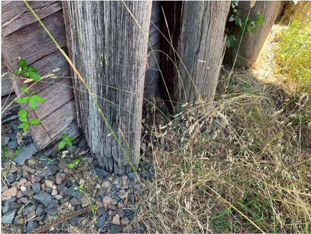
Figure 8-10: View of pile at PB4. Pile was found to be in very poor condition with significant decay present. Decay of approximately 50% of the cross section.
