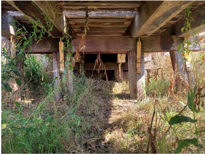
Figure 6-2: View of the typical timber pile bent configuration with each bent varying in height. The bent comprises of 4 driven piles a capsule (cap) and at bent 2 4 corbels located directly underneath girders. Overall, the timber bents were found to be in fair to poor condition. Note: large Wombat hole at abutment 2 between pile 2 and 3 and the significant amount of vegetation growth surrounding the substructure elements. Note that the use of horizontal bolts in the side plates have let to improved pile top condition. Also note the notches in the caps for the girders to drop into.
