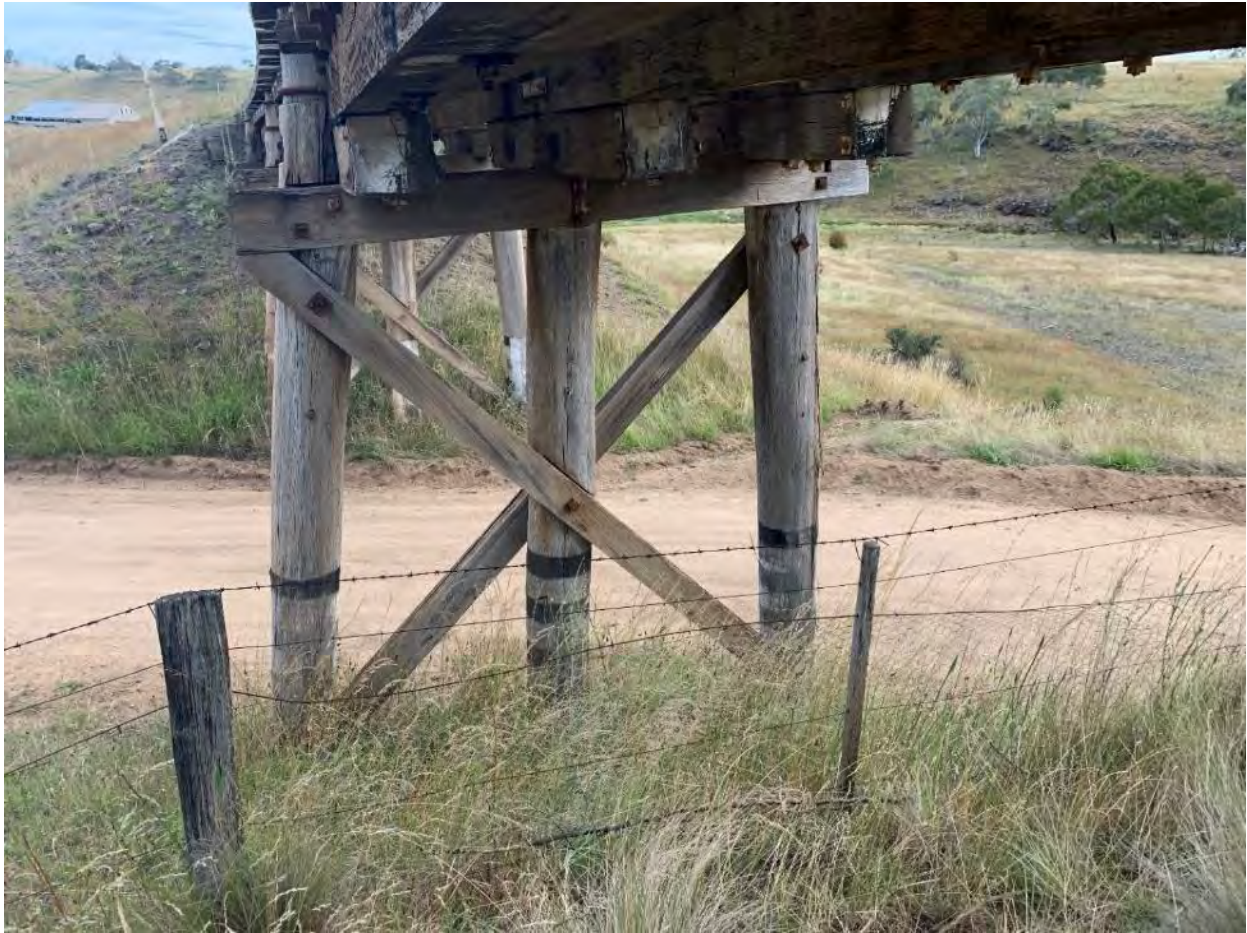
Figure 11-2: View of pile bent 1 configuration. The bents comprise of 3 driven piles. Pile bent 2 and 3 are supported by cross bracing. The two abutments do not contain the cross bracing but are supported by sheeting planks to retain backfill. It was noted that several piles and headstocks have started to undergo decay. It can be seen on pile 3 significant sapwood decay occurring.
