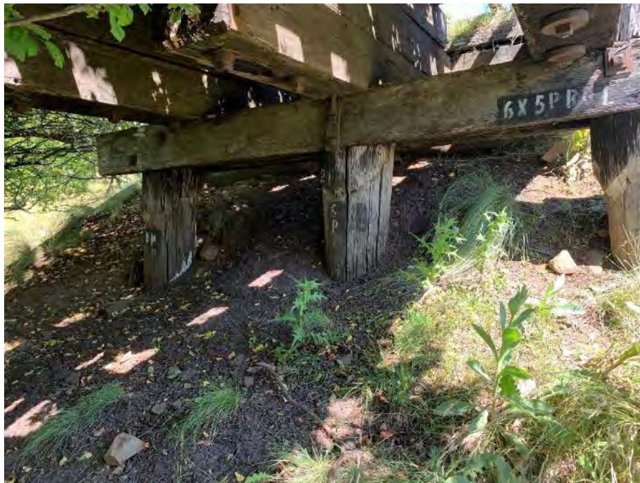
Figure 10-8: View of abutment 2 configuration, the abutment was found to be in poor condition with significant decay present. It was noted that the left two piles had large vertical splits in them, whilst the right pile had significant decay of sapwood.
