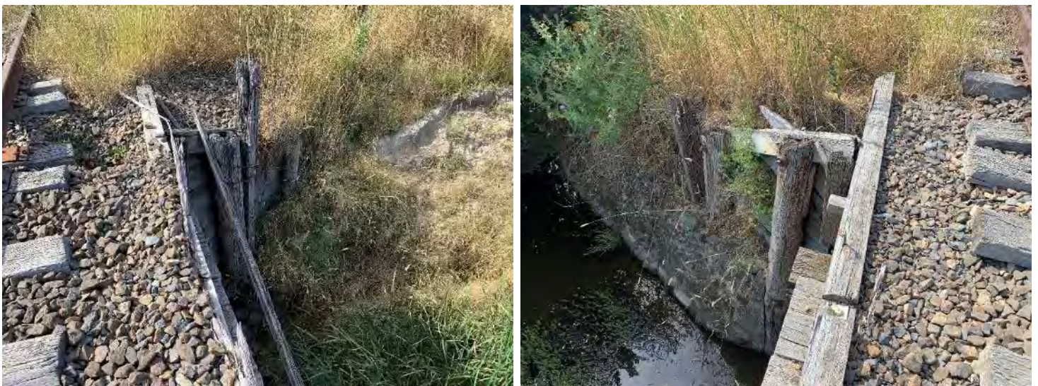
Figure 6-5: Above photos show the existing condition of the wingwalls. The wingwalls were found to be in a poor to very poor condition, multiple members had failed, and significant deterioration was present throughout.
