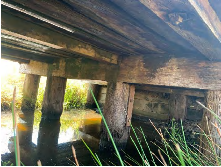
Figure 7-2: Shows the general configuration of the pile bents. Piles are approximately 1m high and in fair condition. Minor deterioration of sapwood is present at water level due to increased moisture content. Water stains and fungal growth present. Note: top plank in abutment sheeting has failed leading to erosion of backfill material.
