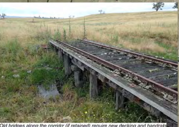
Old bridges along the corridor (if retained) require new decking and handrails
