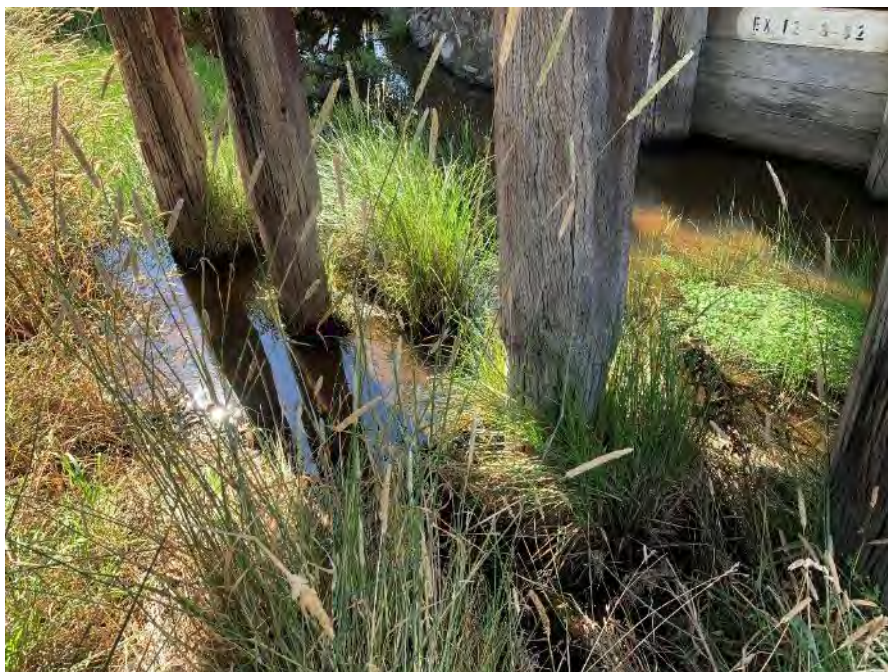
Figure 6-3: A view of Bent 2 shows the timber piles were driven into the creek. Significant sapwood decay is present in the lower length of each pile as seen by the noticeable change in cross section. This is seen as a length that is subject to temporary exposure to moisture which causes accelerated decay compared to constant saturation. Once the moisture content exceeds 22%, timber consuming fungi are activated, and the decay process begins. Refer to Figure 3-2 for a detailed description of how and where the decay occurs due to these vertical bolts.
