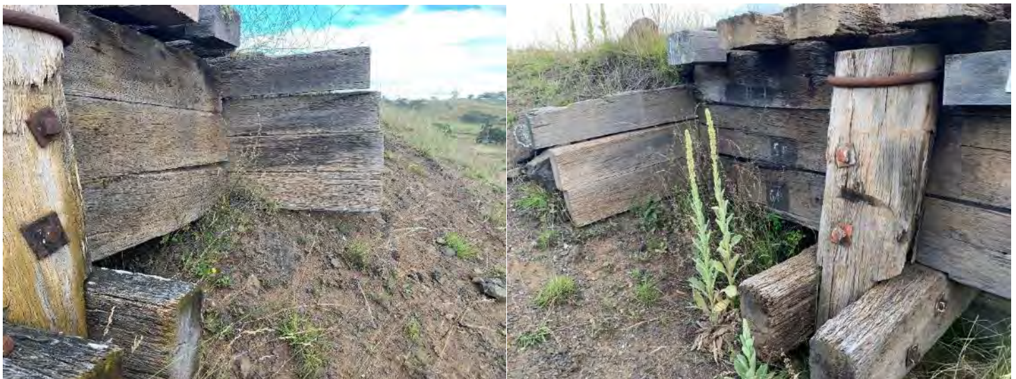
Figure 11-4: The images above show the condition of the breast wall at AB2. The abutment sheeting was found to be in fair condition with minor decay of the sapwood present. The headstock ends were in poor condition with decay and cracking present.
