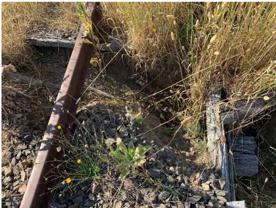
Figure 7-5: Top view of floorboards in the ballast tray at abutment. Large hole caused by abutment/ballast tray failure allowing significant erosion of ballast to occur.
