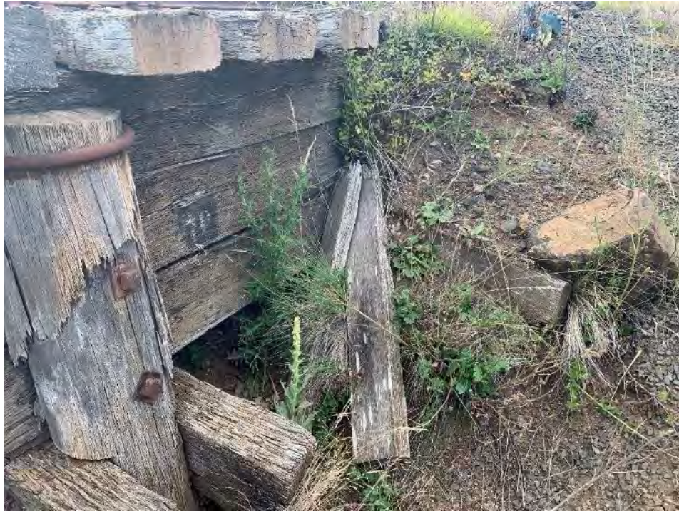
Figure 11-5: View of abutment 1, found to be in poor condition with major decay of sapwood present in piles and broken/missing elements in abutment sheeting.
