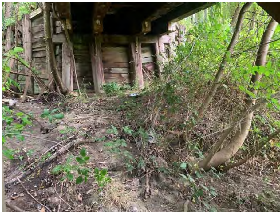
Figure 4-3: Both abutments consist of 4 timber piles, timber headstock, timber corbels and timber sheeting. It was noted that the bottom section of several piles has started to undergo decay. Note abutment sheeting is rotted and failing. Timber pile and sheeting wing walls present on both sides of each abutment. Once the moisture content in the timber elements reaches 22%, decay causing fungi are activated and the decay process begins. Large trees need to be cleared as their root systems apply lateral pressure on the substructure elements as will the branches and trunks on super structure elements.
