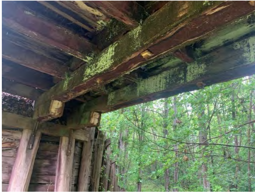
Figure 4-6: View of 2/4 girders. Consists of 4 girder lines which are double stacked with the top girder serving as a lateral bearer beam end stabilizer as well increasing the elevation of the ballast tray floor. All girders exhibited major water stains and decaying fungal growth. Girders were found to be in poor to very poor condition.
