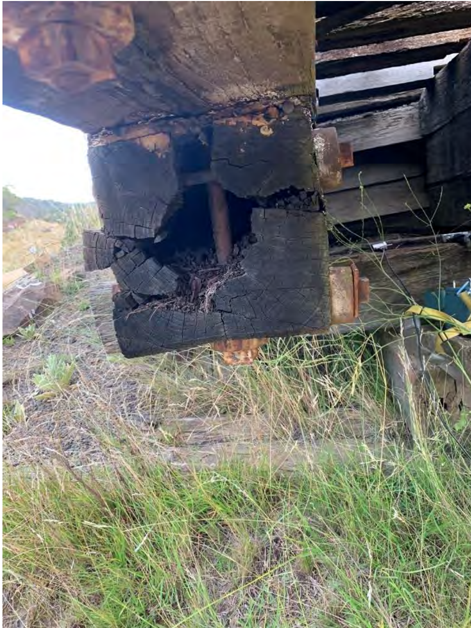
Figure 11-9: View of corbel 3 at abutment 1, Corbel was found to be in very poor condition with a large cavity present in the end. The vertical connection is visible highlighting the depth. The corbel needs replacement due to multiple failure points. Note the vertical fastener has split the corbel and the anti-splitter bolts have done the same thing. So many of these old details contributed to higher maintenance costs and reduced longevity.
