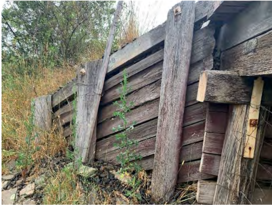
Figure 5-6: A view of abutment wingwall. The wingwall was found to be in fair to poor condition with minor deterioration present throughout all components. Minor deformation was present at top of wall due to bearing load of ballast.
