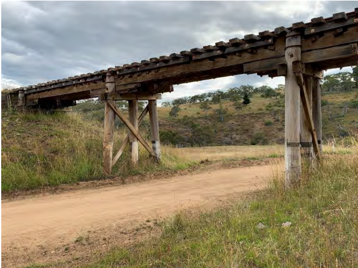
Figure 11-1: General view of Old Bombala Rd Bridge from abutment 1 looking towards abutment 2. The timber bridge is 3 spans long and approximately 22 metres in length (Sp1=7.8m, SP2=6.8m & SP3=6.6m). Note span 2 passes over the road (4.1m Clearance).
