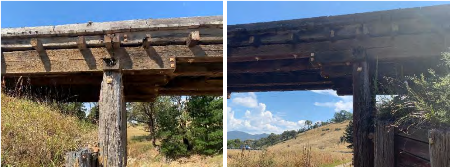
Figure 8-5: View of pile caps at PB1 & 4. Caps were found to be in very poor condition due to the significant cavities present in both ends of each cap. Note: The right photo also shows the backfill from PB4 pushing the breast wall forward.
