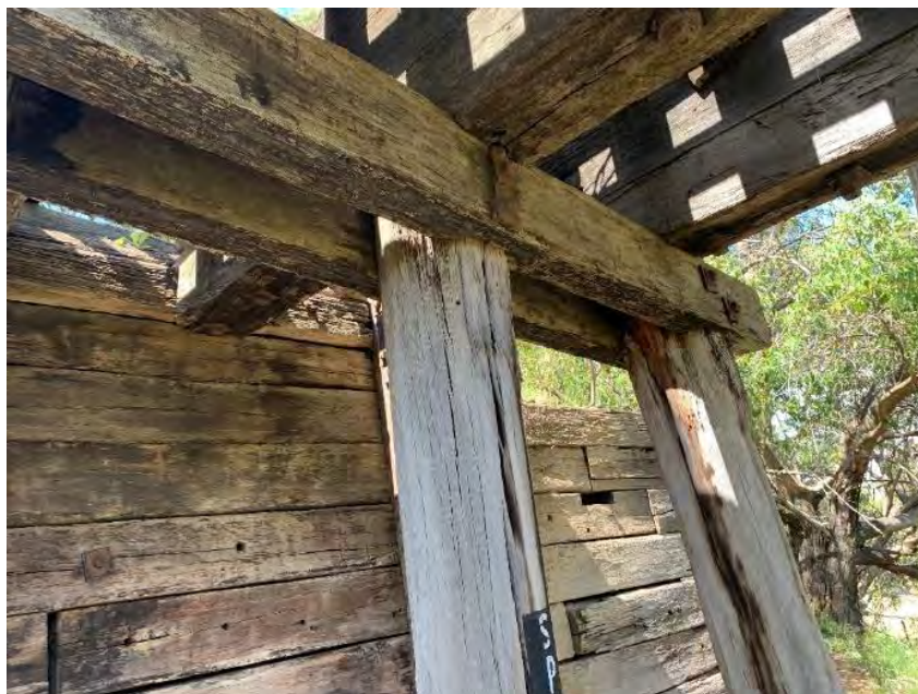
Figure 10-4: The images above show the condition of the split headstocks and the abutment breast wall. The headstocks were found to be in poor to very poor condition, exhibiting significant decay. The breast wall is in poor condition with missing members and weathered elements with splits and cracking throughout. Note: major vertical crack down middle pile exposing bright wood and accelerating decay. Typically, these decay cracks are initiated by fastener systems
